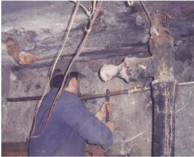
Repairing water supply works in multi-apartment buildings- Community-Based Urban Water Supply Management Contract
